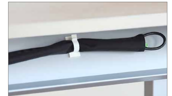
Cable conduit for stowing the cables in the cable duct
